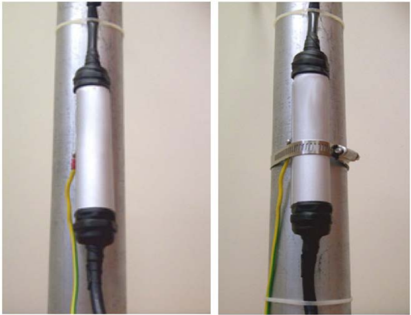
Figure 3-35: Mounted and strapped to the pole
